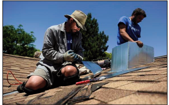
Photo by Cyrus McCrimmon, The Denver Post Tim Steele, left, and Bowen Christensen with The Cooler Company Heating & Air install an evaporative cooler on the roof of a home in Wheat Ridge.
