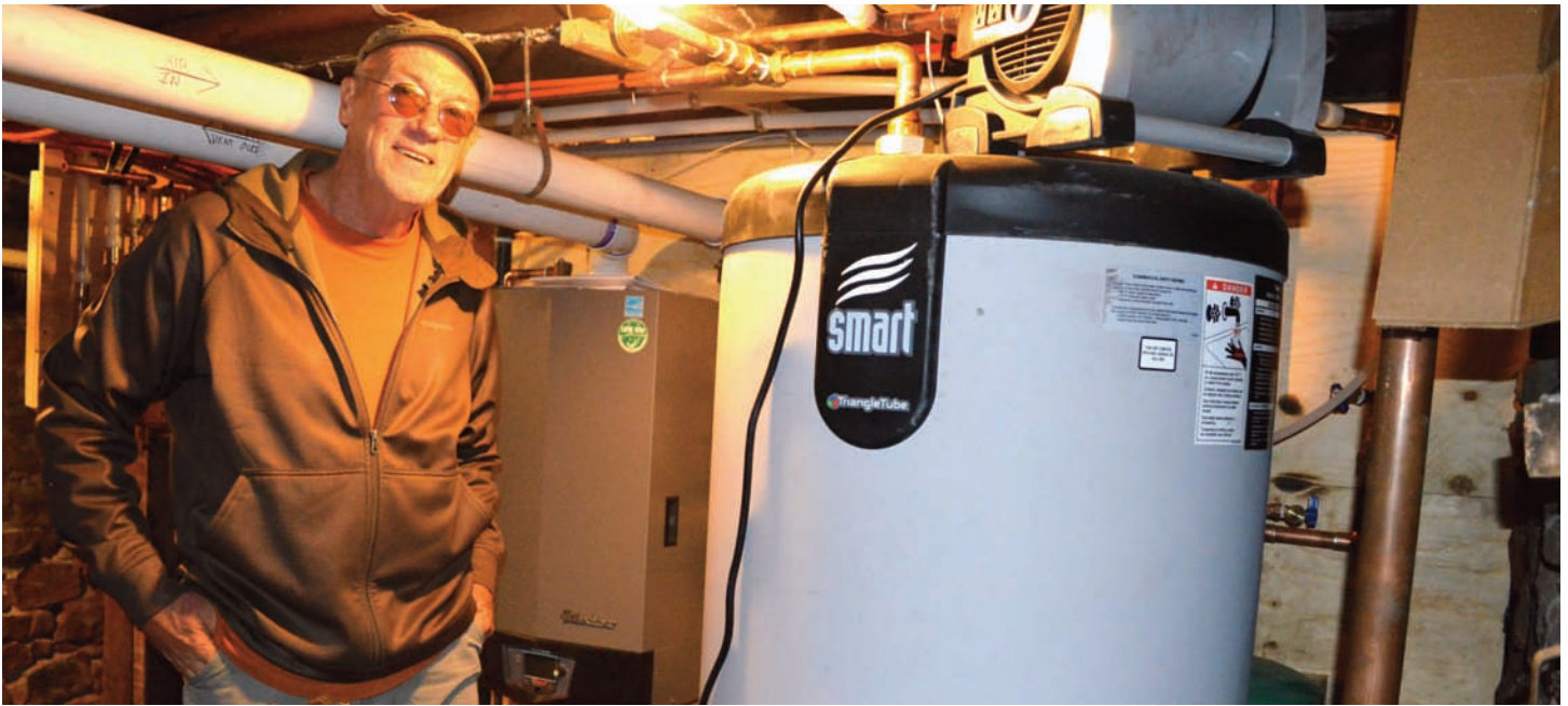
Above: John Ackerman shows off the new boiler and hot water tank (with heat exchanger) in the Pink Palace's basement.
